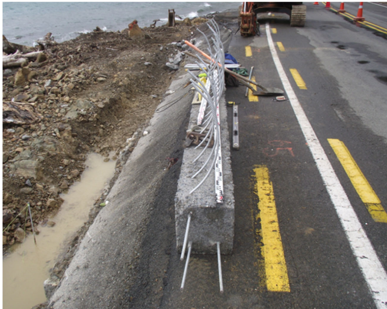
Figure 2-7: Shallow excavations and reinforcing at York Bay. [Source: Design Features Report (Stantec 2018b)].
