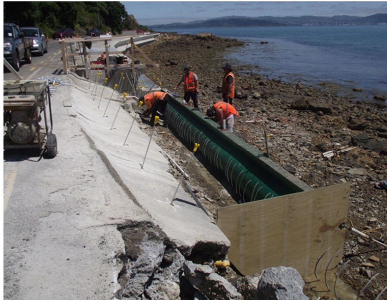
Figure 2-8: Example of in situ construction methodology at York Bay. [Source: Design Features Report (Stantec 2018b)].
