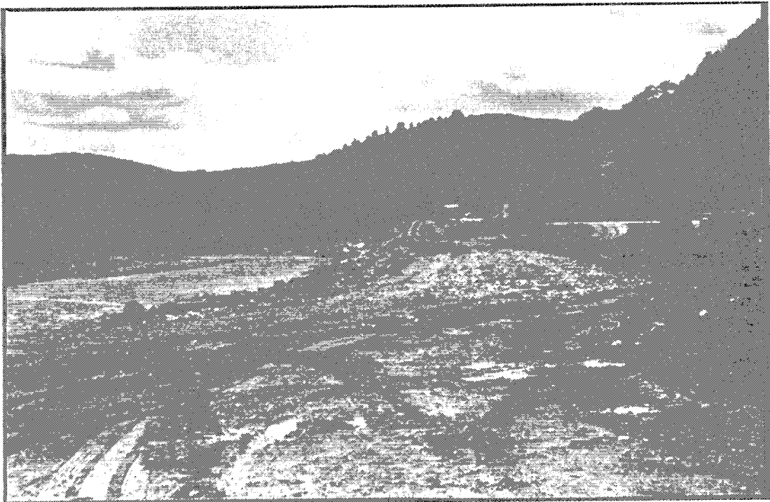
Plate 97: Hutt River bed south of the Mangaroa confluence at the start of highway construction. The river flowed against the highway before the diversion.
